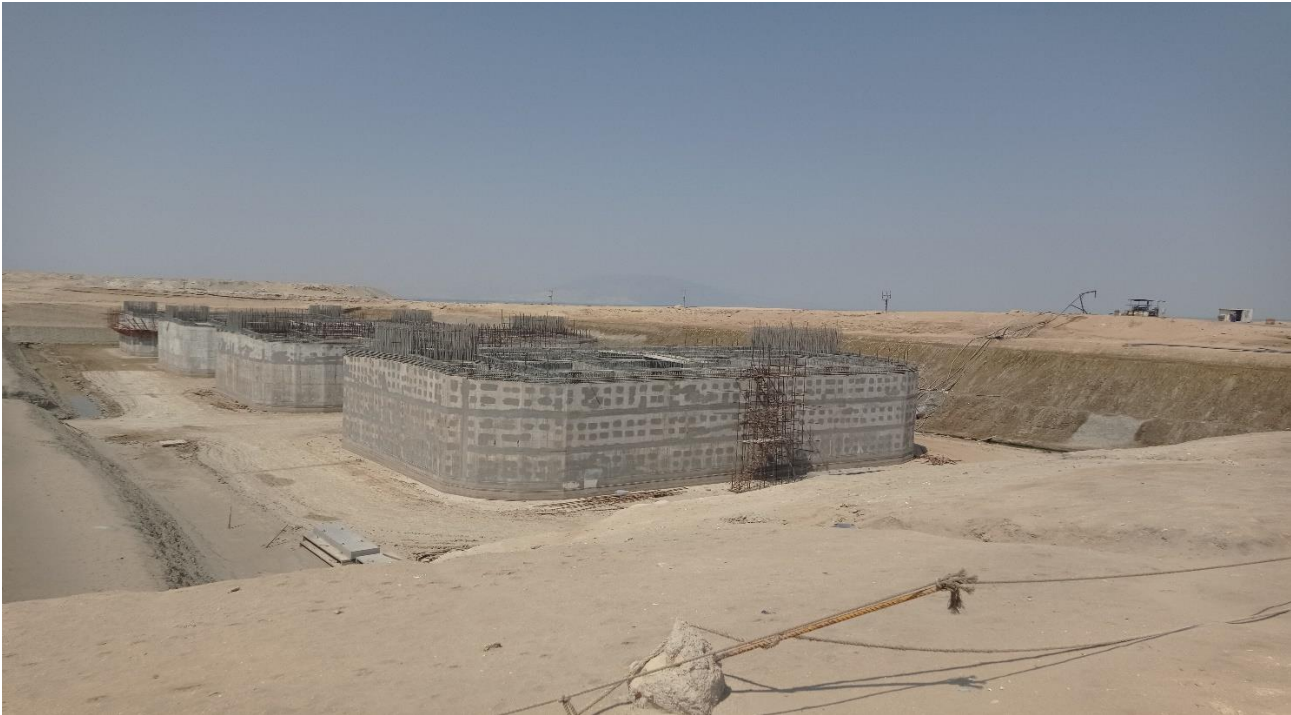
Figure 8 Working area to build the Persian Gulf bridge in Qeshm Island, October 2023. Credits: SpecialEurasia
